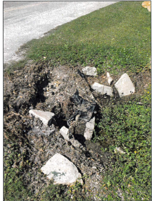
Clogged Culvert (Myrtle St.)
