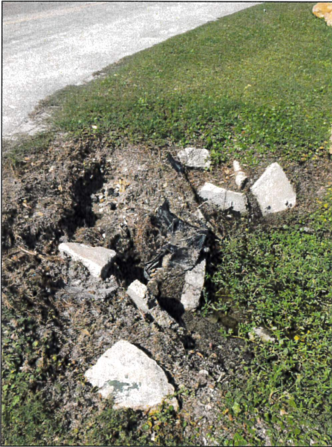
Clogged Culvert (Myrtle St.)
