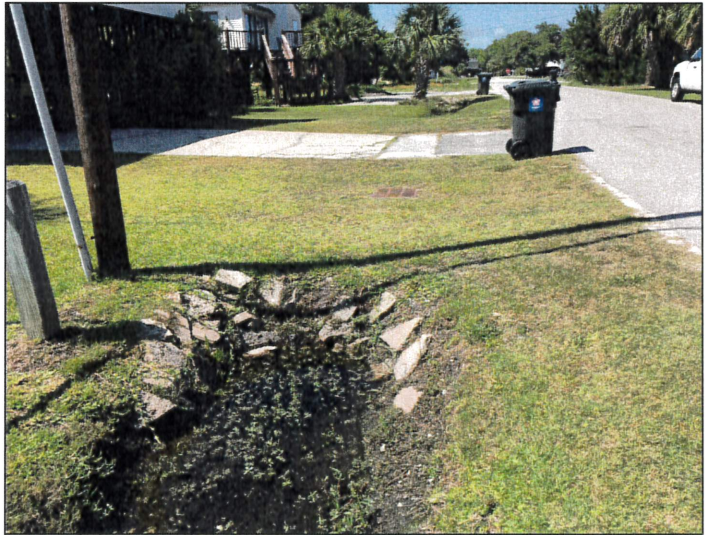
Standing Water along Billow St.
