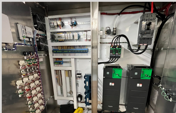
Upgraded control panel at Pump Station A
